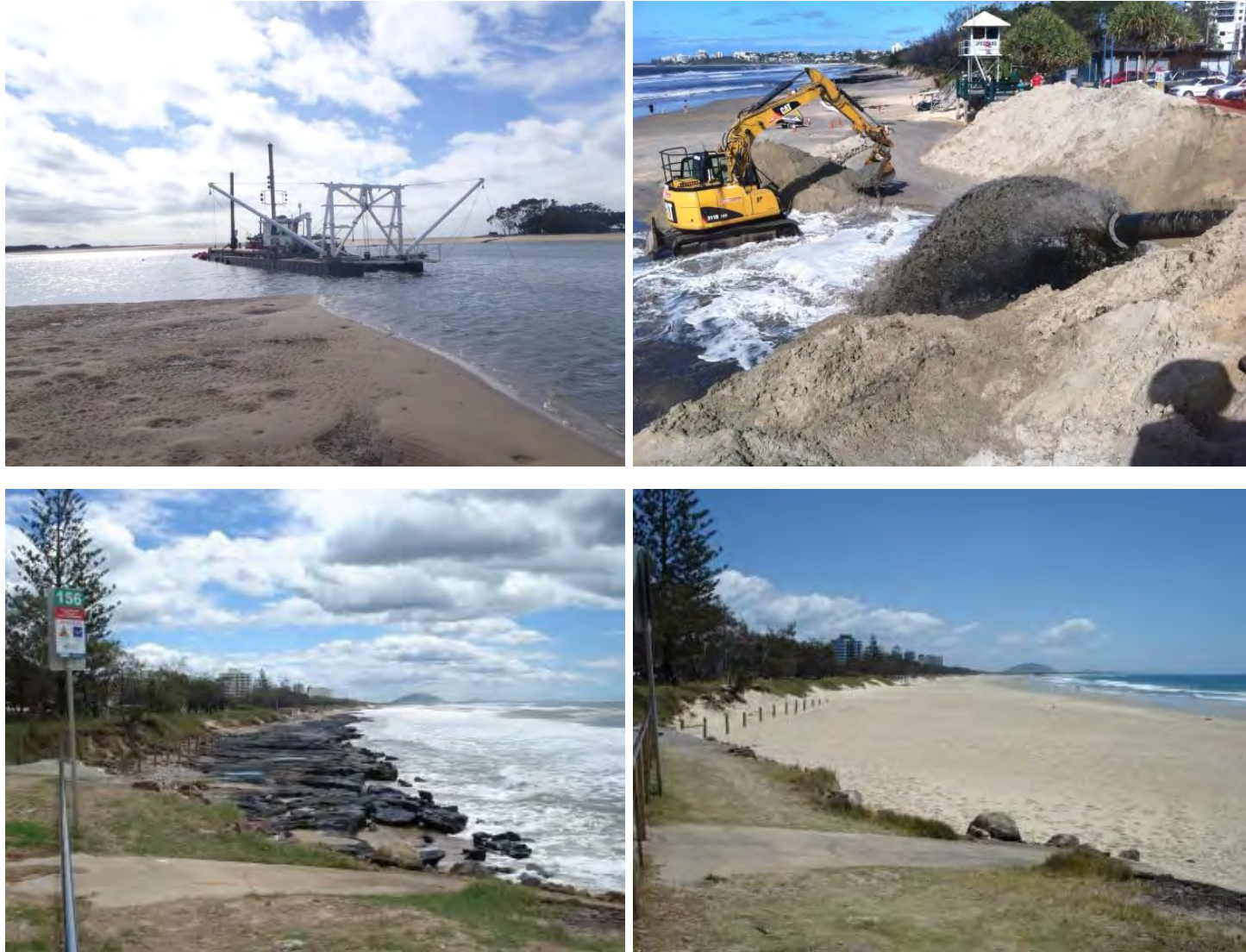
Figure 3-2 Stage 1 Dredging and Nourishment (clockwise from top left): Birdon Pty Ltd CSD Dogo in the Lower Maroochy River; Sand Delivery to Maroochydore Beach; Beach Condition after Nourishment Works; Beach Condition before Nourishment Works
